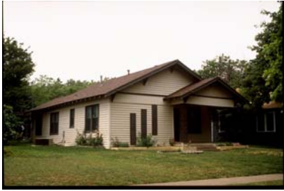
METAL SIDING with CHANGES AT WINDOWS and LOSS of MAJORITY OF TRIM
