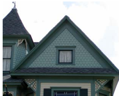
TRIM AT A QUEEN ANNE HOUSE: GABLE TRIM, WINDOW TRIM, FINIAL AT ROOF, TEXTURED SHINGLES AT GABLE and DECORATIVE CORNER BRACKETS.
