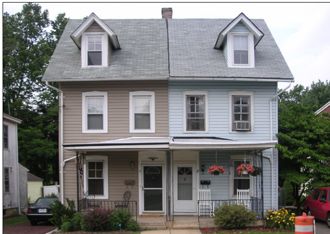
Vinyl siding of different colors has been installed at each residence. The siding is not aligned and obscures wood window surrounds.
