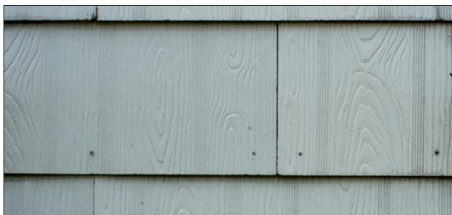
Asbestos siding is often embossed with a wood grain pattern. The removal of asbestos siding can be dangerous and should be undertaken by trained professionals.
