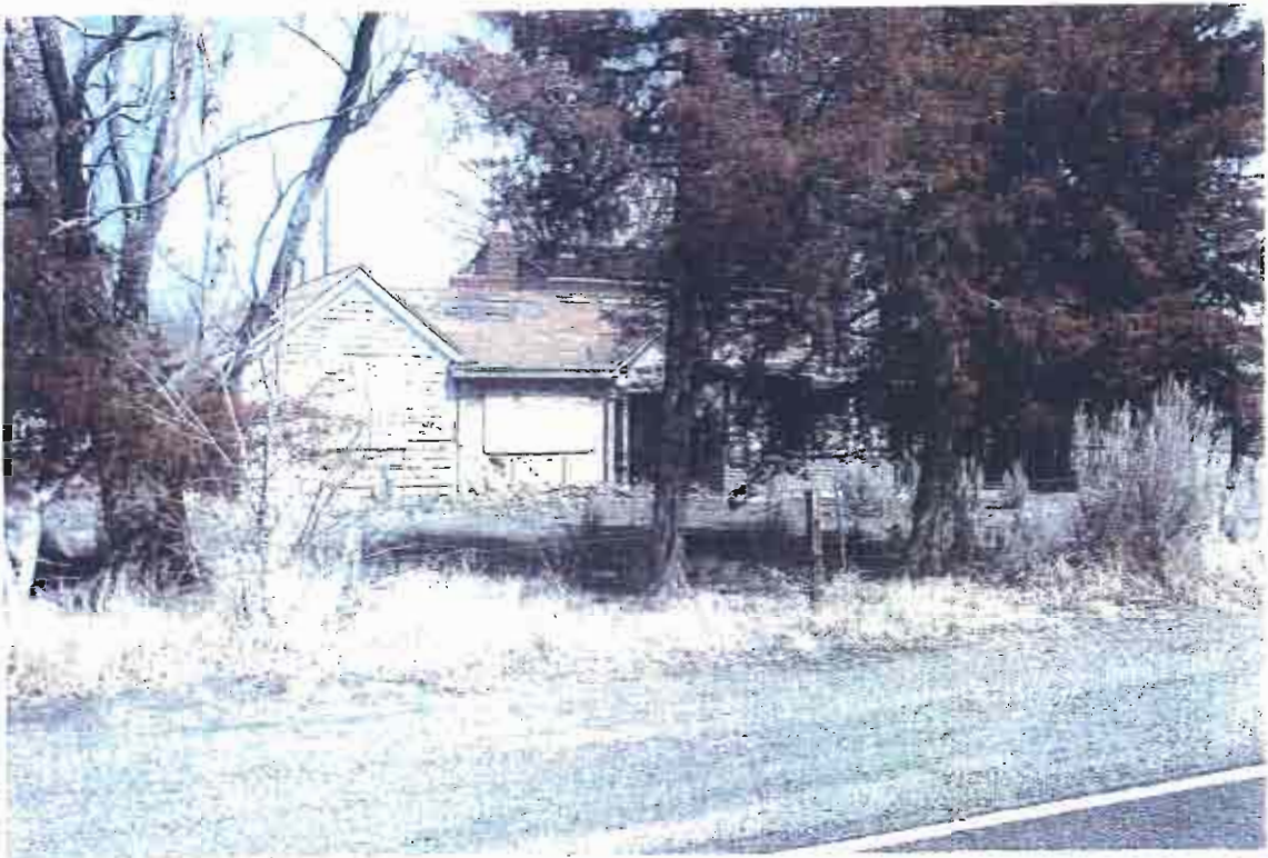
Deteriorating dwelling in the ranchyard.
