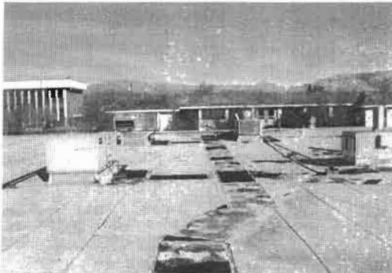
Another overall view of roof system, very dry roof. This roof needs to be restored or replaced very soon !!!!
