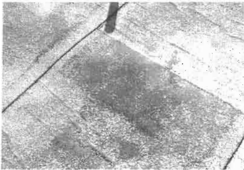
Granulars have lost adhesion from cap sheet, UV and water will accelerate the deterioration of the material
