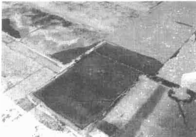
Existing walk pads are deteriorated or missing
