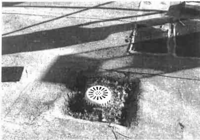
Lots of debris around internal drains
