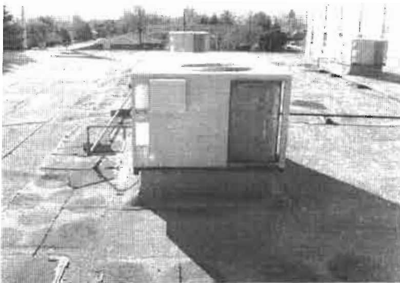
View of HVAC units, nice high curbs on these units
