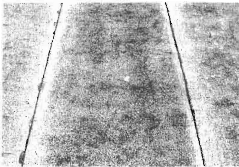
Granular loss on entire system
