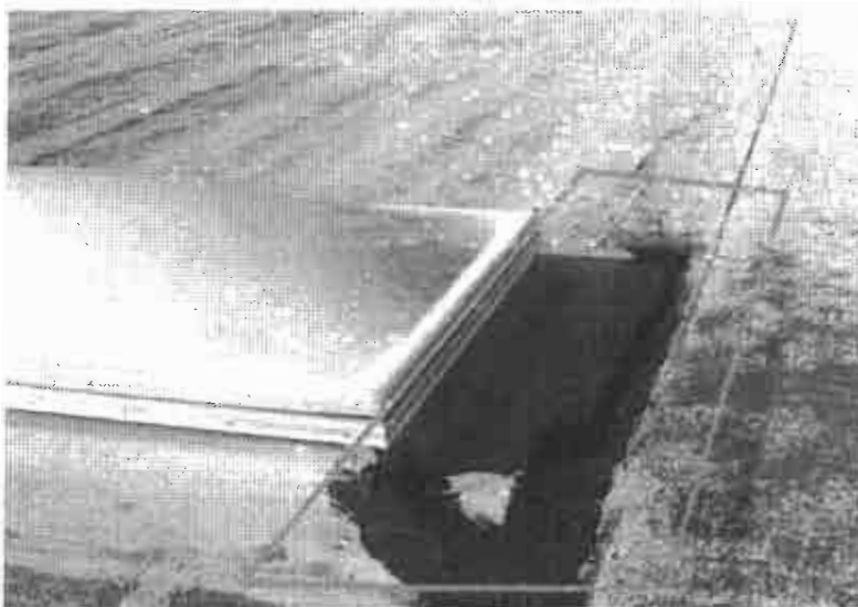
Previous failed repair, black mastic should not be used when repair is exposed to UV. A silver reflective fiberized mastic is the proper material...
