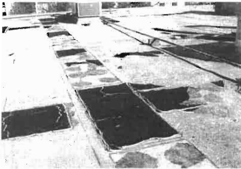
All walk pads are deteriorated and/or missing
