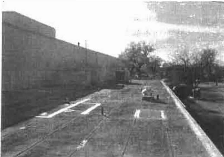
View of lower overhang section of roof system, notice granular loss on mineral cap sheet
