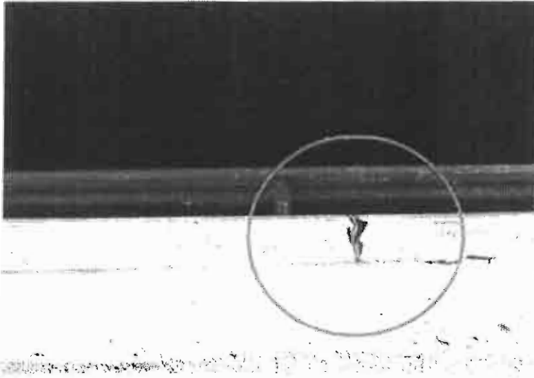
Damage at all seams on edge metal, the existing mineral cap sheet is not strong enough to with stand the expansion and contraction of the metal
