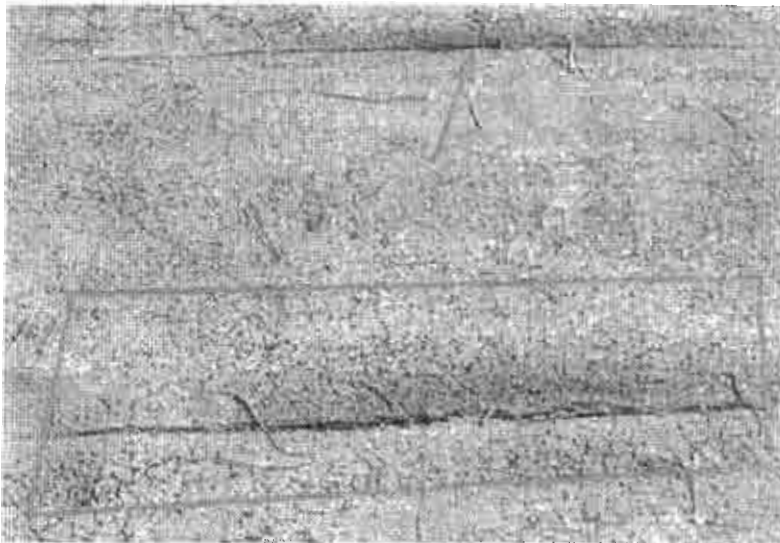
Blisters in roof system, this is a result of moisture in the roof
