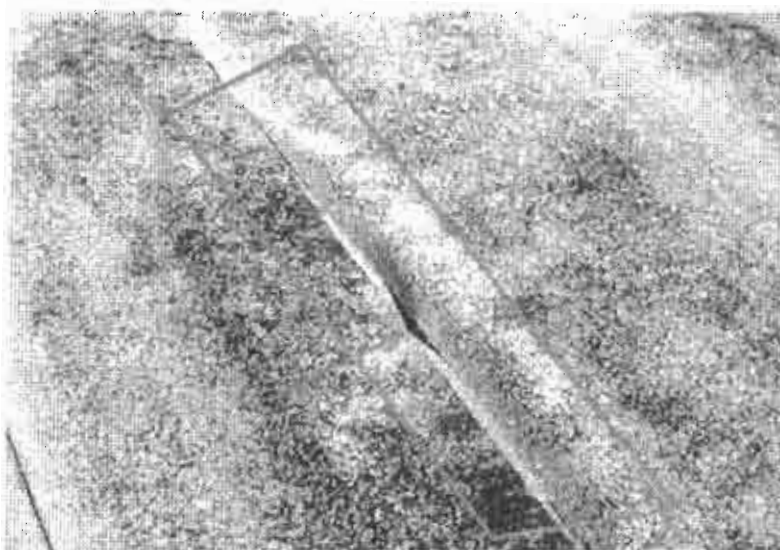
Seam separation and blisters in roof system. The blister is formed when water enters roof system and water vapors damage inter plies of roof
