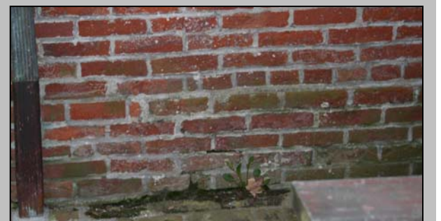
Moisture is the most significant cause of decay in masonry. Seen here are examples of spalling, efflorescence, and organic growth, all caused by excessive moisture.
