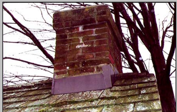
Deterioration that is not addressed can compromise the effectiveness and soundness of your roof system.
