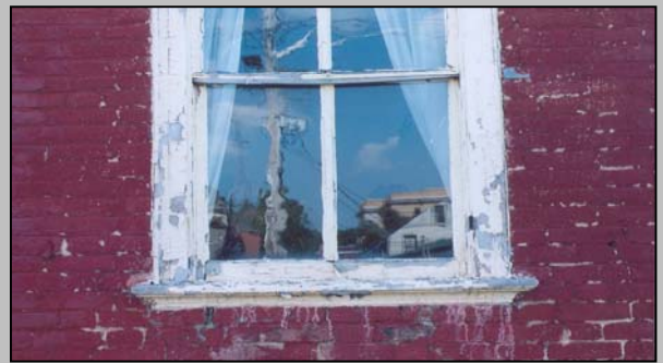
To ensure a long operating life, windows should be regularly maintained, and deterioration should be addressed before it compromises the structural stability and efficiency of the unit
