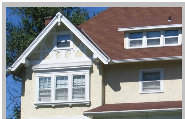
These exterior storm windows are perfectly fitted with the historic windows so that the meeting rail on the storm window aligns with that of the historic window. In addition, the trim color and scale is appropriate for the window openings
