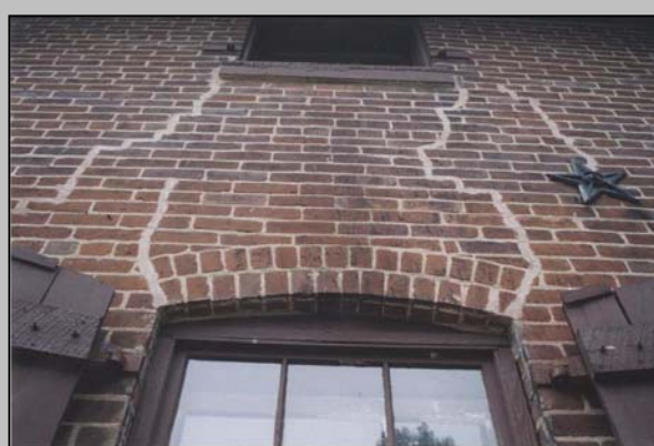
Cracks that have settled and have been inspected by a professional can safely be patched, but they should be patched in a manner that does not detract from the historic masonry
