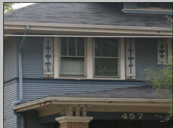
Shutters should only be installed where they were historically found. They should also be installed as a functional building element that covers the entire window opening, not simply as a decorative element as they are on this house.
