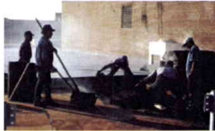
The first ply of hot applied, built-up roofing is installed over perlite insulation board. The system is carefully installed to accommodate locations of roof penetrations and rooftop mechanical equipment. (Photograph courtesy of Wiss, Janney Elstner and Associates)
