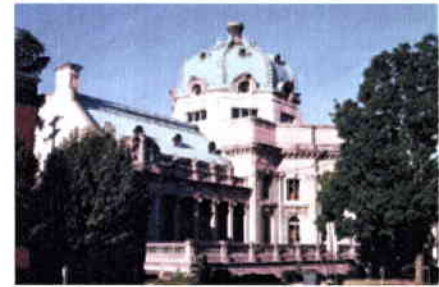
Copper was put to effective use on the roof of the 1913 Handley Library in Winchester, Virginia. (NPS photo) [click image for larger view]
