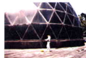
This investigator is using a nuclear moisture meter to identify areas of moisture in the roof system. The nuclear moisture meter is most appropriate for use with gravel surfaced built-up,
