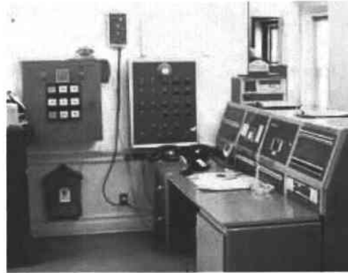
Complex mechanical systems for institutional buildings may require a central control room. Photo: NPS files.
