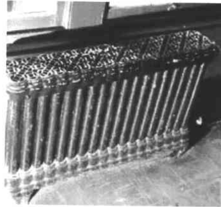
This radiator would be identified as a significant element of the interior. In any work to upgrade the mechanical system, it would be retained and preserved, even if non-functioning. Photo: NPS files.
