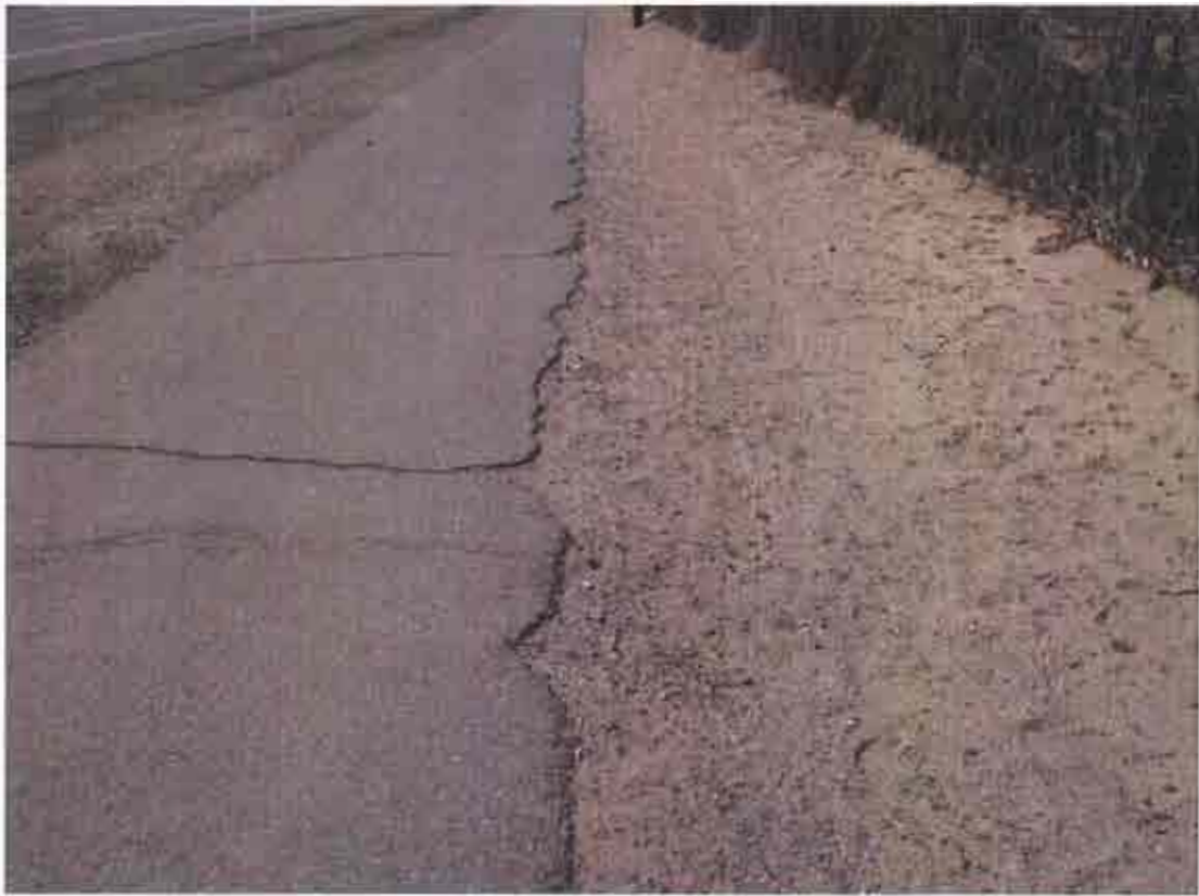
Asphalt Deterioration Along Edge of Path
