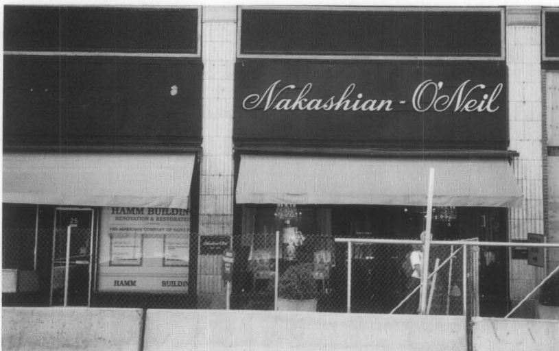
Figure 4. When the Hamm Building rehabilitation began, most of the prismatic tiles (above the awnings) were hidden beneath plywood panels. Photo: Oertel Architects.
