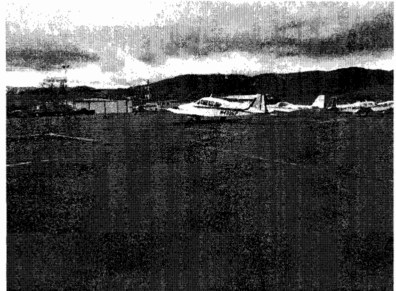
Typical vegetation in cracks on the main apron
