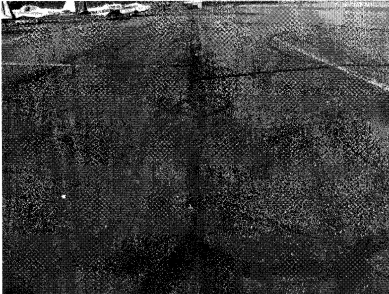
Typical alligator cracking on a pavement joint
