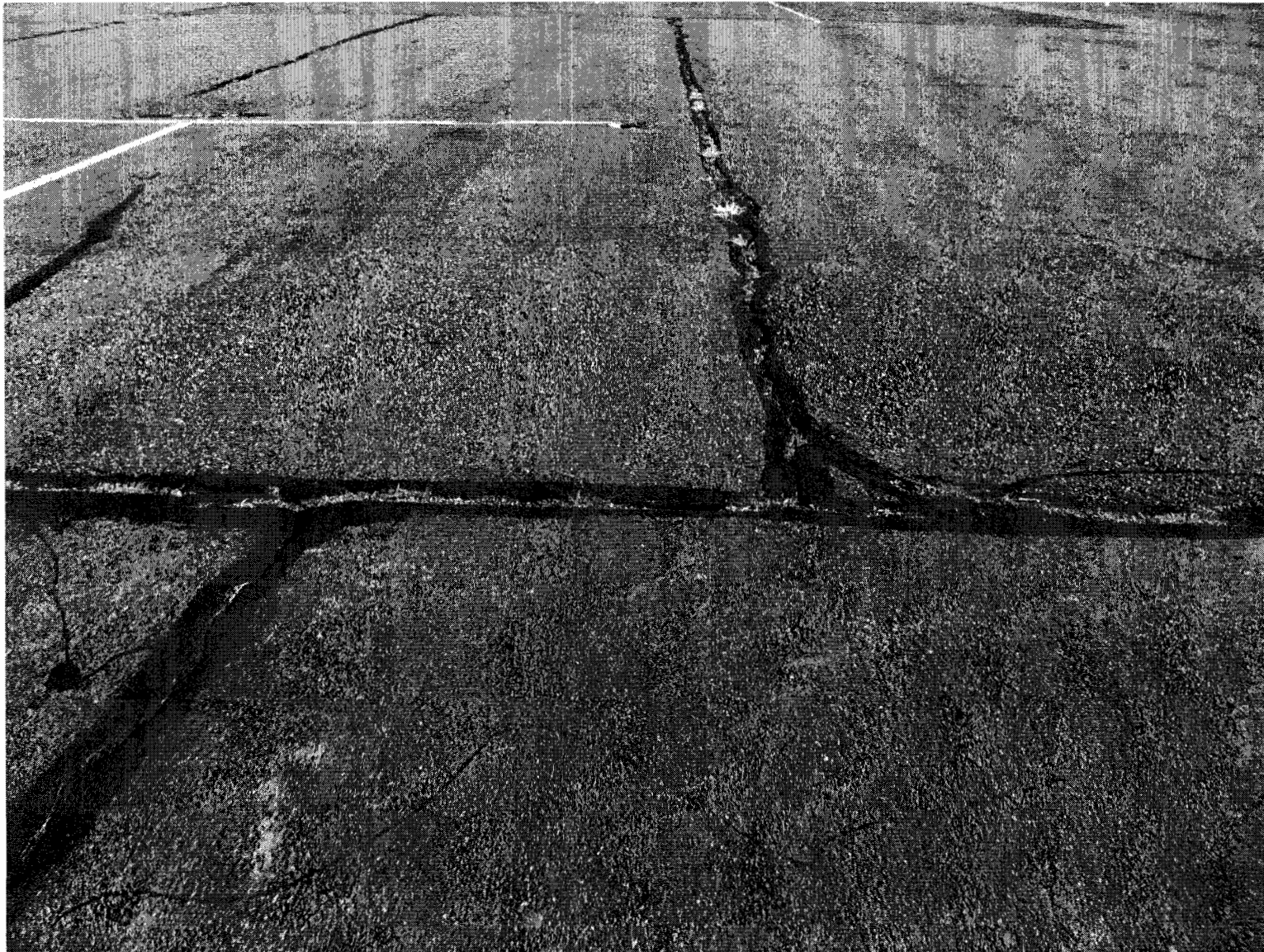
Point #5 showing typical cracking and spalling in Phase 3 of the reconstruction of the main apron
