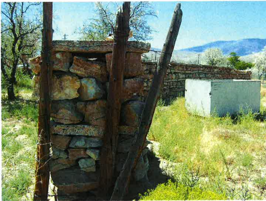
Figure 6. East and North Side of Rock wall adjacent to WRF view West.
