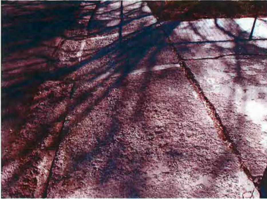
Sidewalk Deterioration/Non ADA-Compliant Drive Access
