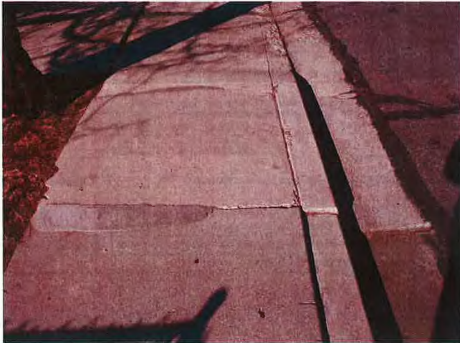
Insufficient/Temporary Patch on Sidewalk Heaving
