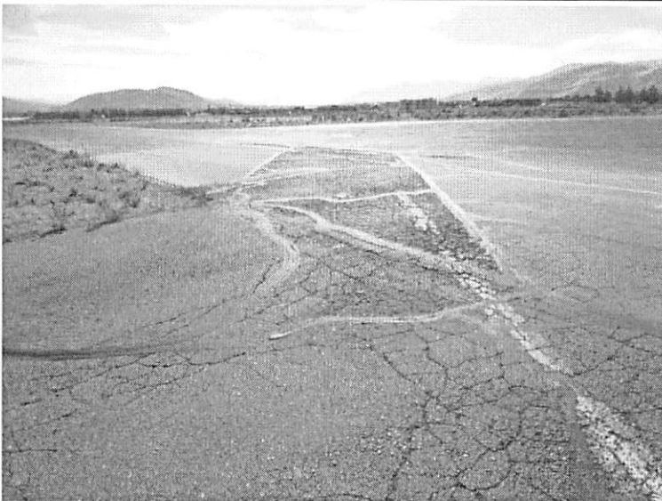
Failing pavement patch through the main taxiway to Taxiway D
