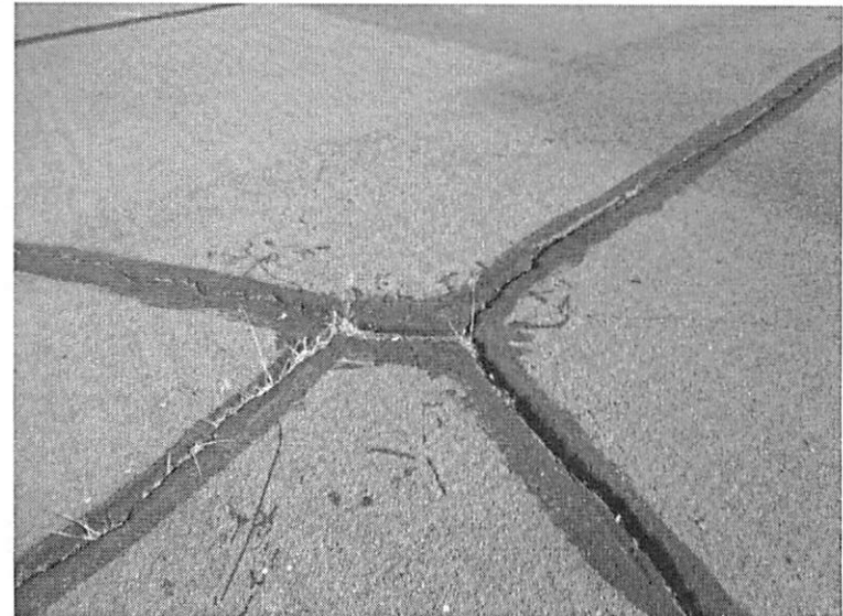
Typical cracking in the north apron pavement
