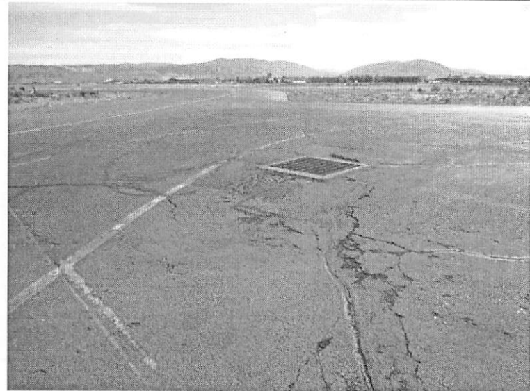
Inadequate drainage feature at the main taxiway to Taxiway D
