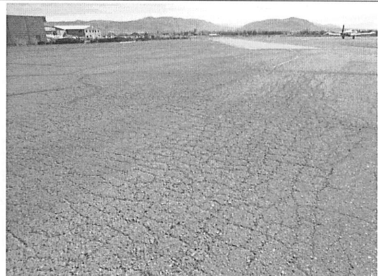
Alligator cracking in the main taxiway in the north apron
