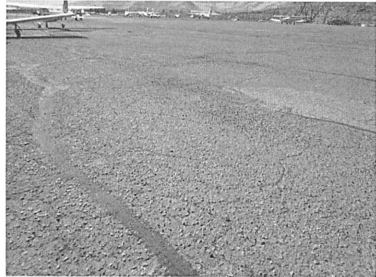
Typical raveling/alligator cracking near the main taxiway in the north apron
