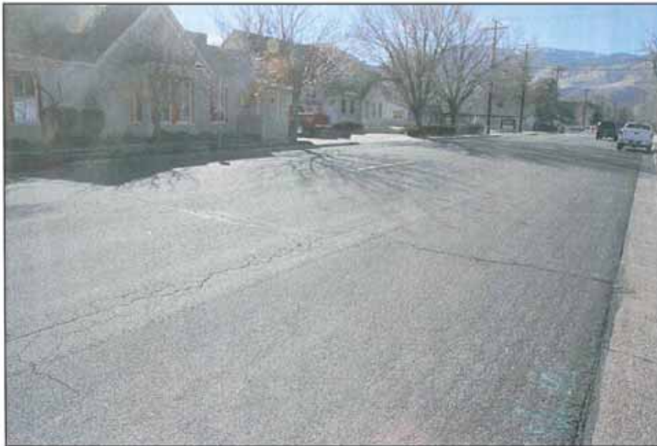
Photograph #9 View facing west from NW corner of N. Curry St. towards N. Nevada St. showing chip seal surface and existing transverse and longitudinal cracking w/ alligator cracking as well.
