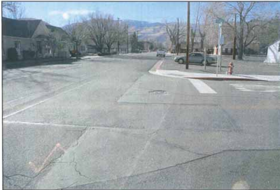
Photograph #6 View looking west of patching and cracking in west bound lane at N. Curry St. looking towards N. Division St.
