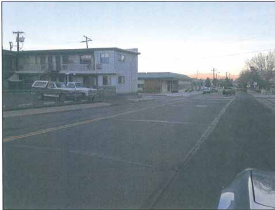
Photograph #11 View facing east from Carson Street towards Plaza St. showing cracking and patching.
