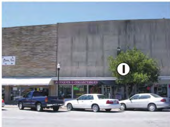
① The use of light gauge metal, steel panels, or other materials to make two or more storefronts appear to be a larger structure should be avoided.
