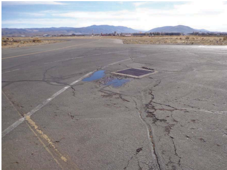
Inadequate drainage feature at the main taxilane to Taxiway D
