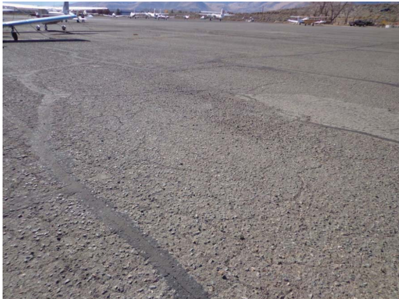
Typical raveling/alligator cracking near the main taxilane in the north apron
