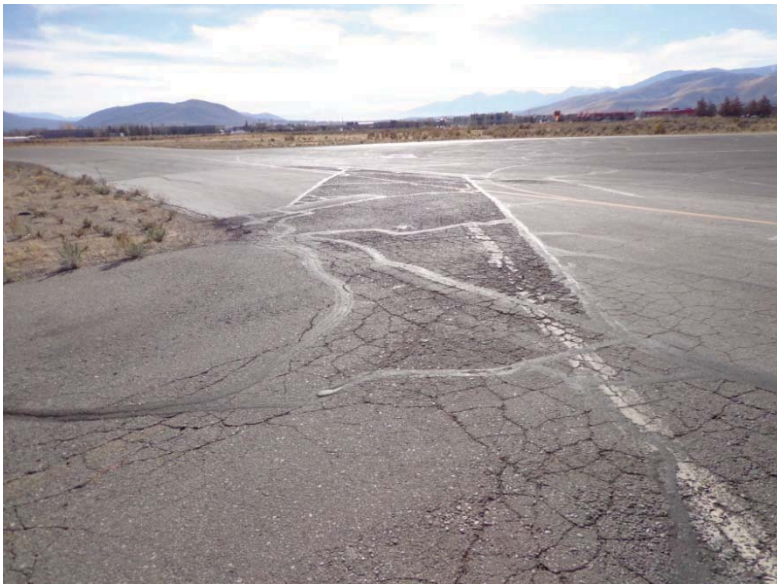
Failing pavement patch through the main taxilane to Taxiway D
