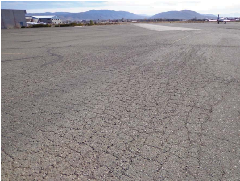
Alligator cracking in the main taxilane in the north apron
