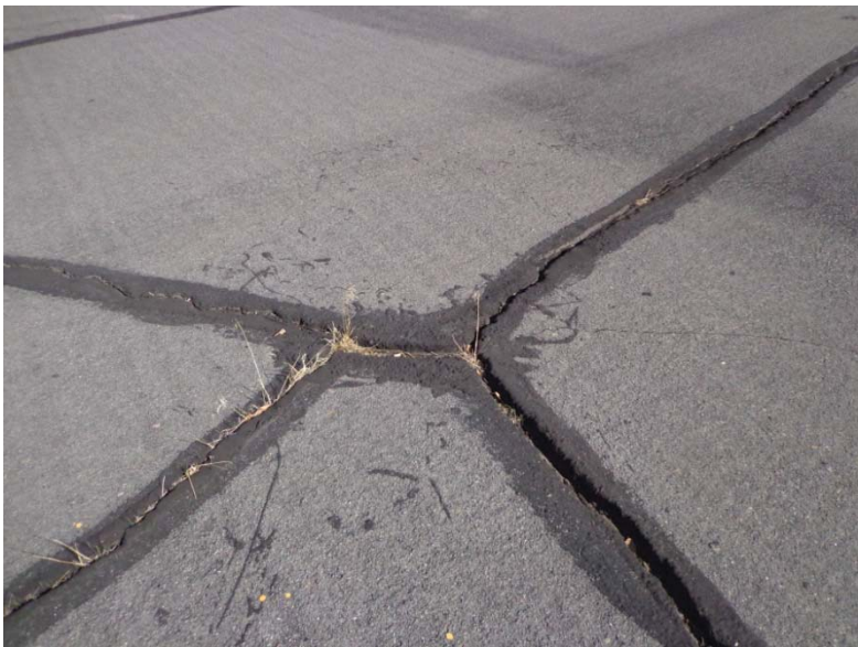
Typical cracking in the north apron pavement
