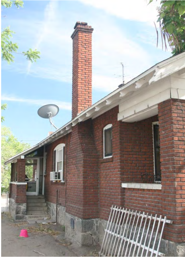
Figure 19. Unreinforced masonry residence. The home is built on an inhomogeneous rubble-rock foundation, is likely not tied to the foundation, is made of ridged brick that break apart with strong earthquake forces, and has a topple hazard, the tall chimney. Possible secondary hazards include gas leaks and fire if the gas meter or hoses are damaged or further damaged by aftershocks. Shelter would likely be required for the residents following a major earthquake.
