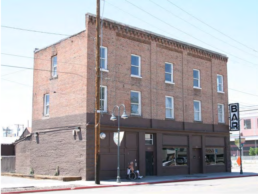
Figure 20. Unreinforced masonry commercial building with an unsupported parapet and crowning bond beam. The wheelchair-bound man below would have a difficult time getting out of the way during the shaking from an earthquake.
