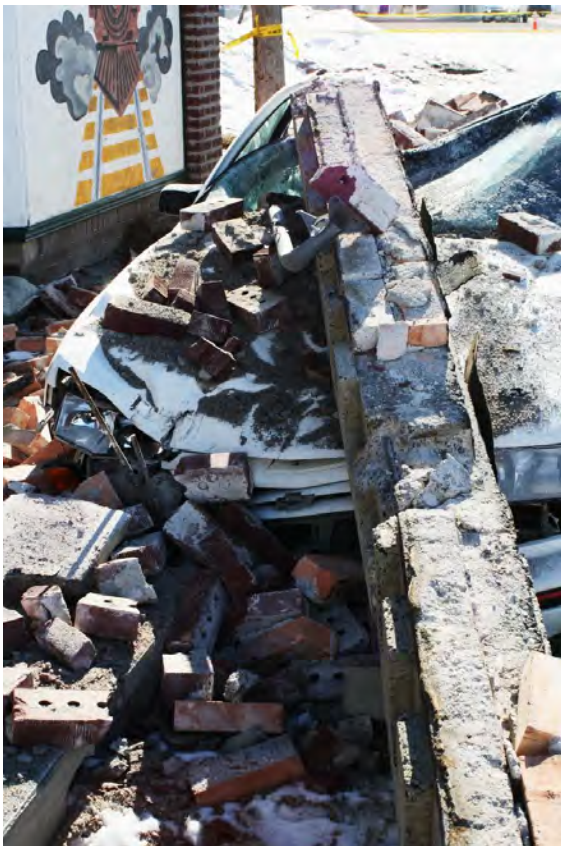
Figure 21. Bricks and crowning bond beam that fell on a car during the 2008 Wells, Nevada earthquake. Unreinforced masonry buildings can shed debris like this on sidewalks, alleys, and other buildings around them.
