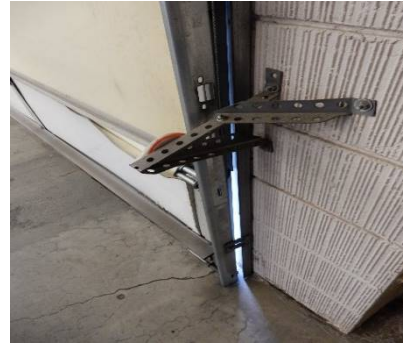
Fire Station 52 damaged Weather-Stripping
