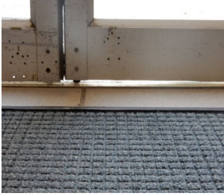
Community Center Damaged Vertical Sweep
