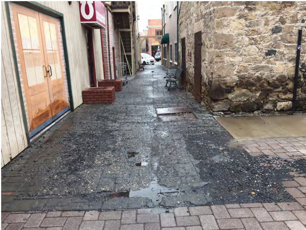
Deteriorating concrete and benches
