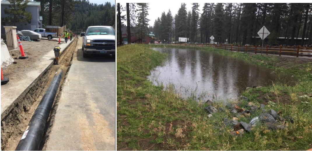
Zephyr Cove GID Water Quality Improvement Project: Left, installation of storm drain, Right, Newly constructed basin collecting runoff.
