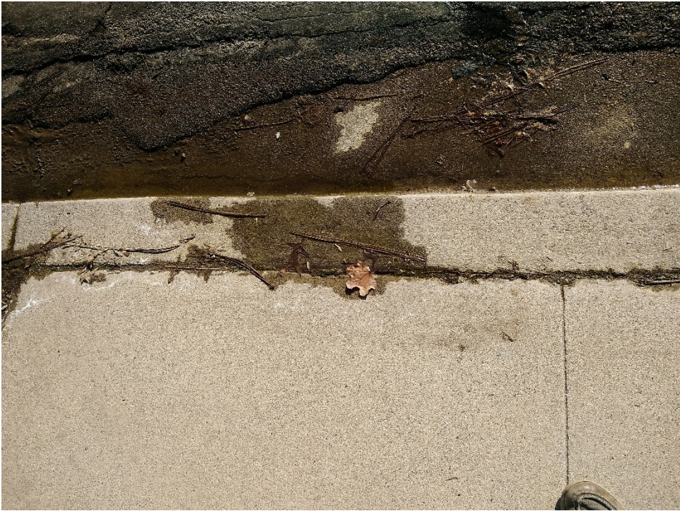
Water coming up through sidewalk at driveway:
