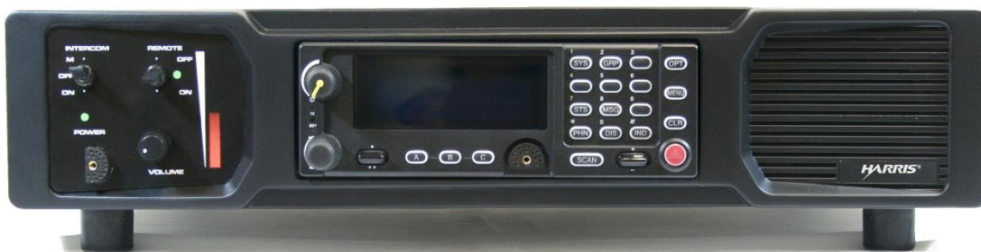
Figure 3. NDOT’s NSRS Control Station Configuration
