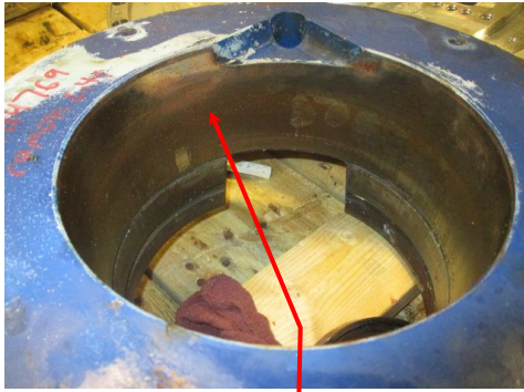
Effluent End Bearing Housing
