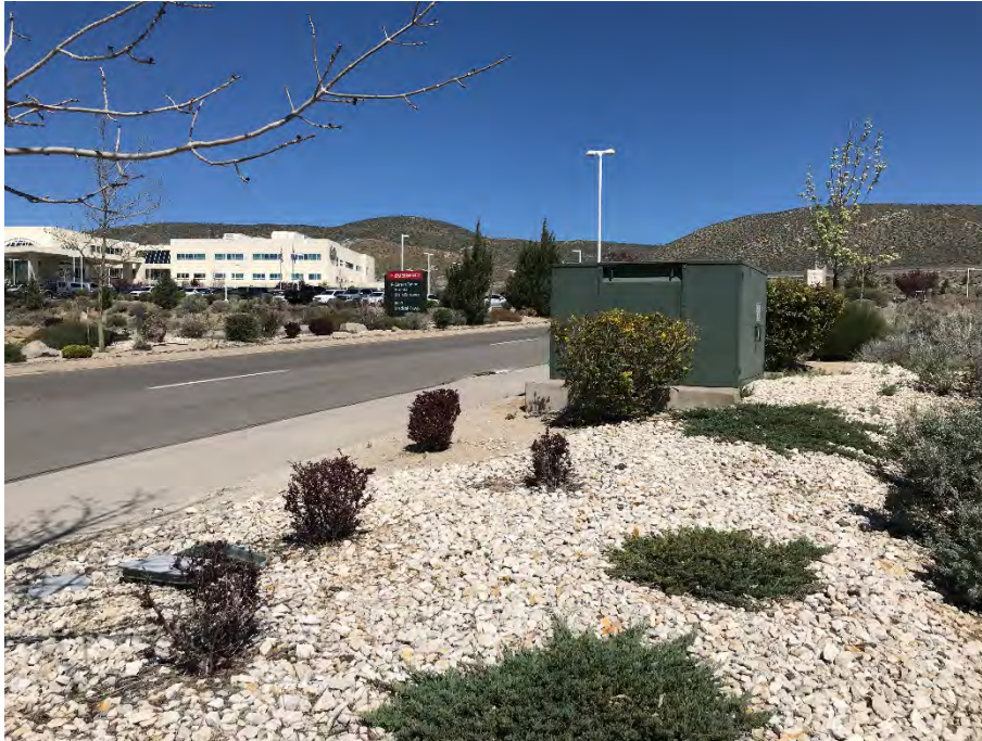
Photograph 3: View a transformer located on the western Property boundary.
