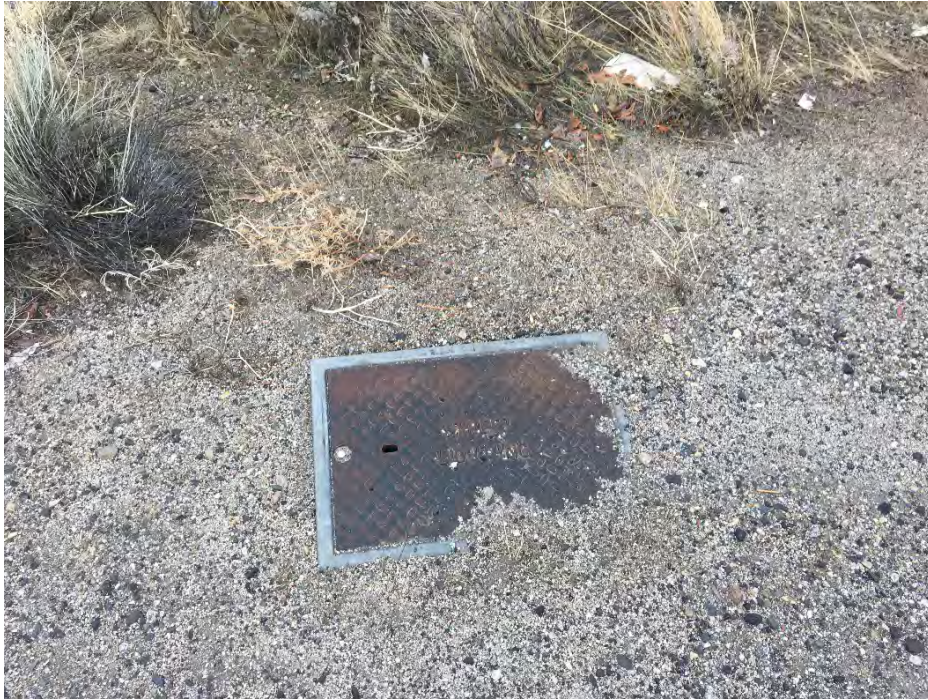
Photograph 9: Electrical connection for future street lighting along Butti Way.
