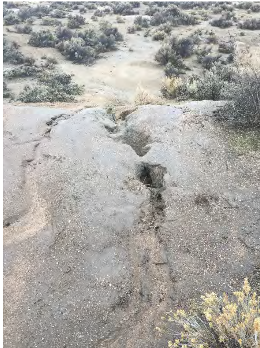
Photograph 4: Evidence of soil fissures on southwest corner of the Property at the intersection of Butti Way and Airport Road.
