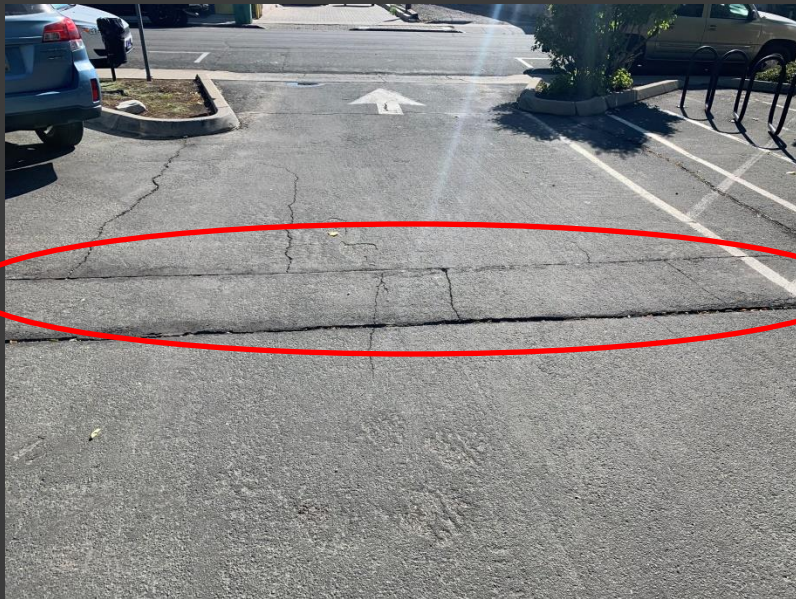
Failed Pavement Sections
