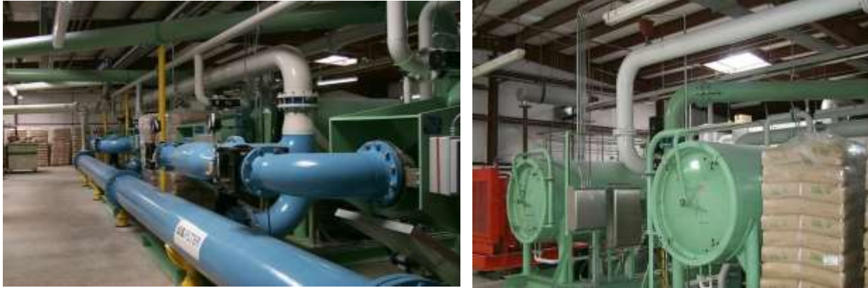
Quill Water Treatment Plant
