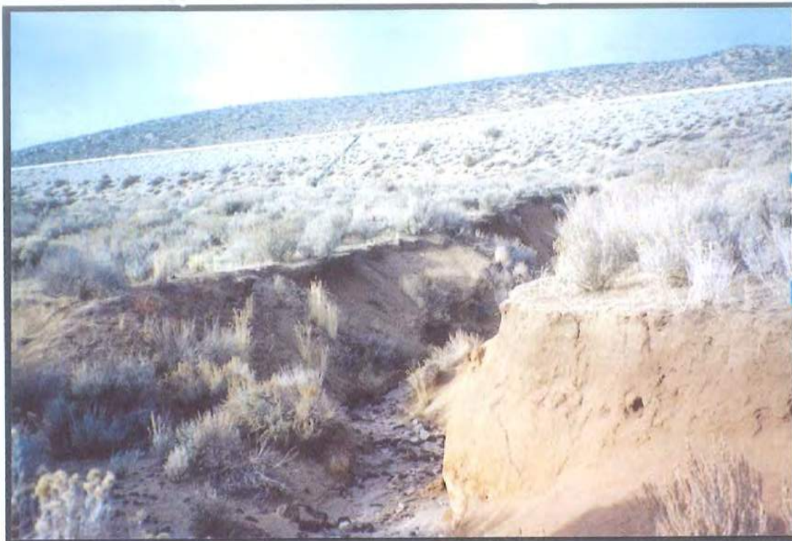
PHOTO 5. CHANNEL ERODED BY ROAD RUNOFF FROM HIGHWAY 395. PIPE CONVEYING RUNOFF FROM HIGHWAY VISIBLE ON ROAD-FILL SLOPE.
