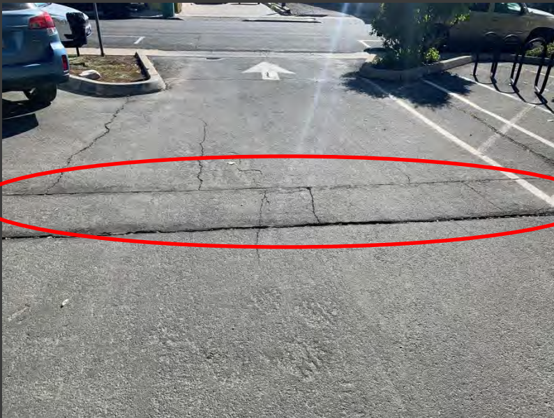
Failed Pavement Sections
