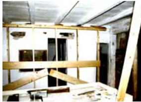
Interior bracing which will last the duration of the mothballing will protect weakened structural members. Photo: John Milner Architects.
