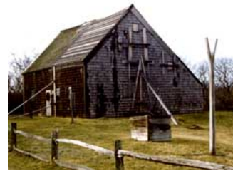
Buildings seriously damaged by storms or deterioration may need to be braced before architectural evaluations can be made. Photo: John Milner Architects. Photo: NPS files
