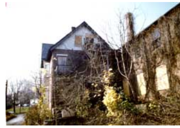
Boarding up without adequate ventilation and maintenance has accelerated deterioration of this property. Photo: NPS files.
