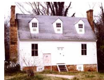
Regrading has protected this masonry foundation wall from excessive damp during its 10-year mothballing. Note the attic and basement vents, temporary stairs, and interpretive sign. Photo: NPS files.
