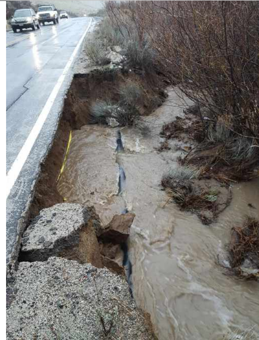
Roadside Damage Due to Flooding in 2017
