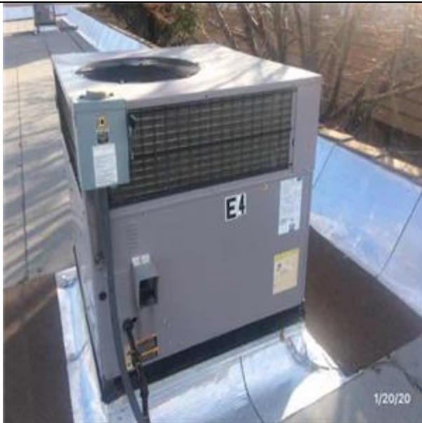
View of Packaged Rooftop A/C With Heat, Under 20 Tons - E-4
