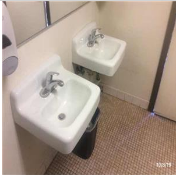
D2013 Lavatories :- View of Wall Hung Lavatories
