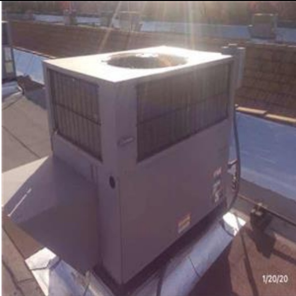
View of Packaged Rooftop A/C With Heat, Under 20 Tons - E-11
