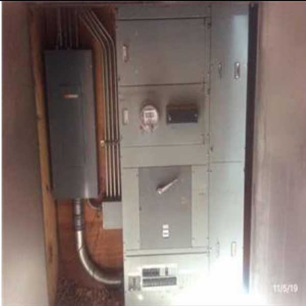
View of Switchboard - 120/208volts, 400 to 2000amp
