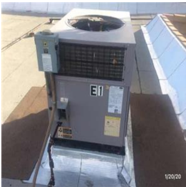
View of Packaged Rooftop A/C With Heat, Under 20 Tons - E-1
