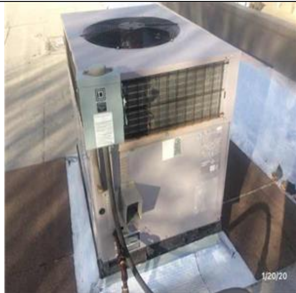
D3052 Package Units :- View of Packaged Rooftop A/C With Heat, Under 20 Tons - E-5
