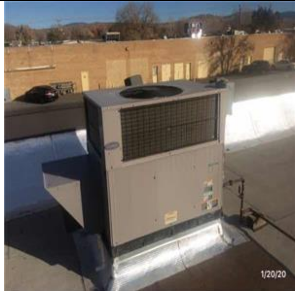
D3052 Package Units :- View of Packaged Rooftop A/C With Heat, Under 20 Tons - E-12
