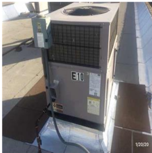
D3052 Package Units :- View of Packaged Rooftop A/C With Heat, Under 20 Tons - E-10
