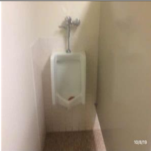
View of Wall Hung Urinals
