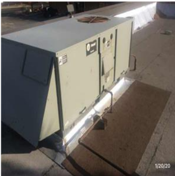
View of Packaged Rooftop A/C With Heat, Under 20 Tons - E-2
