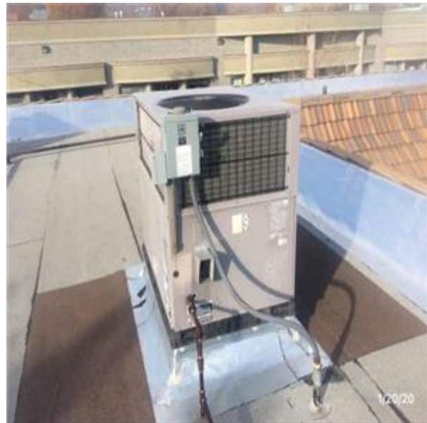
D3052 Package Units :- View of Packaged Rooftop A/C With Heat, Under 20 Tons - W-9
