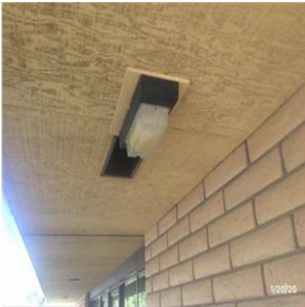
View of Exterior Wall Pack Light Fixtures
