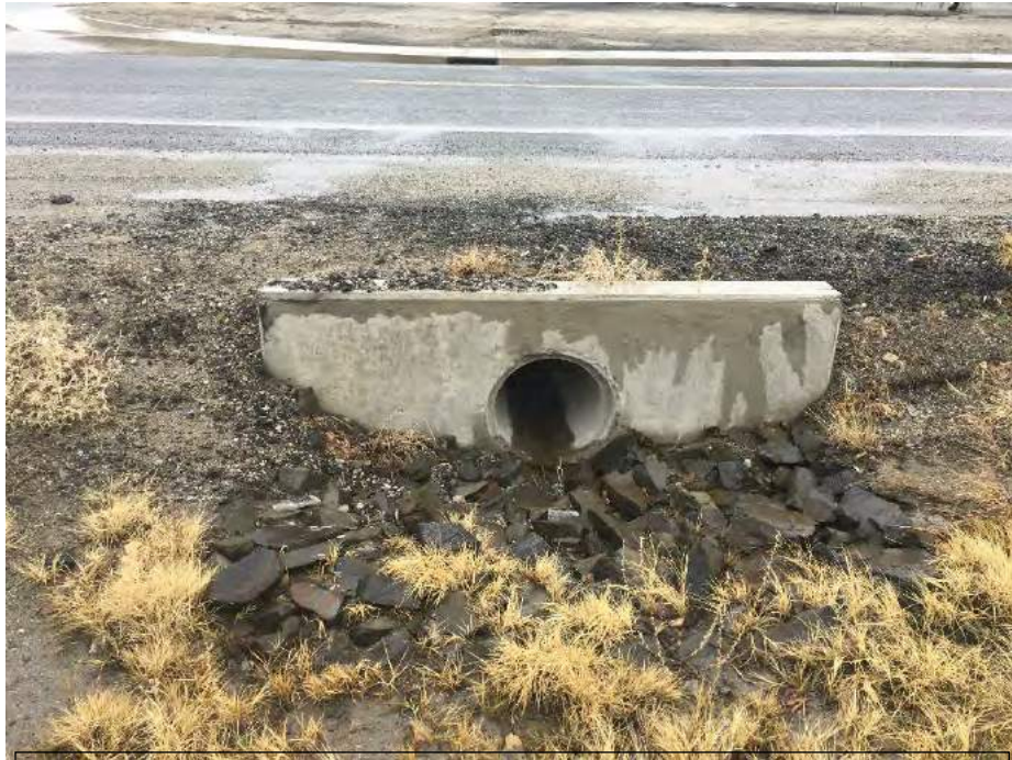
Picture 11: Drainage ditch running under Butti Way north to south in central portion of the Property.
