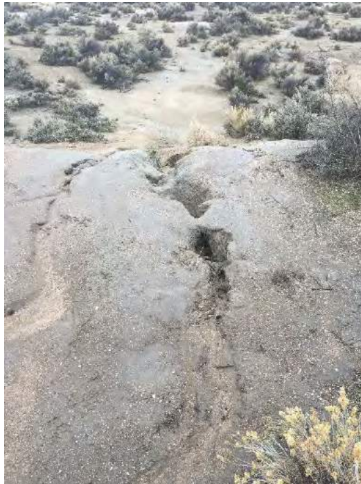
Photograph 4: Evidence of soil fissures on southwest corner of the Property at the intersection of Butti Way and Airport Road.
