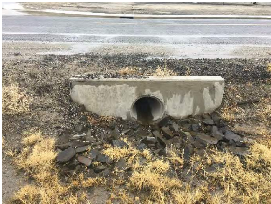
Photograph 6: Drainage ditch running under Butti Way north to south in central portion of the Property.
