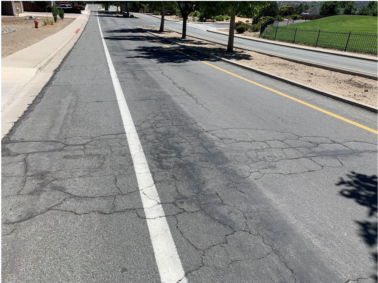
Figure 5. Pavement in Poor condition category (PCI 55-41).
