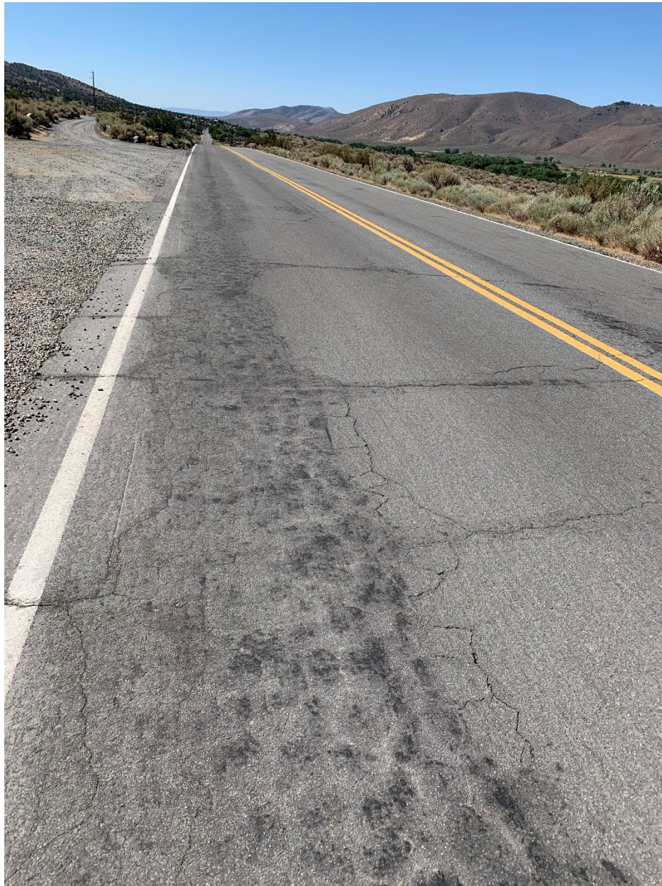
Figure 7. Pavement in Serious condition category (PCI 25-11).
