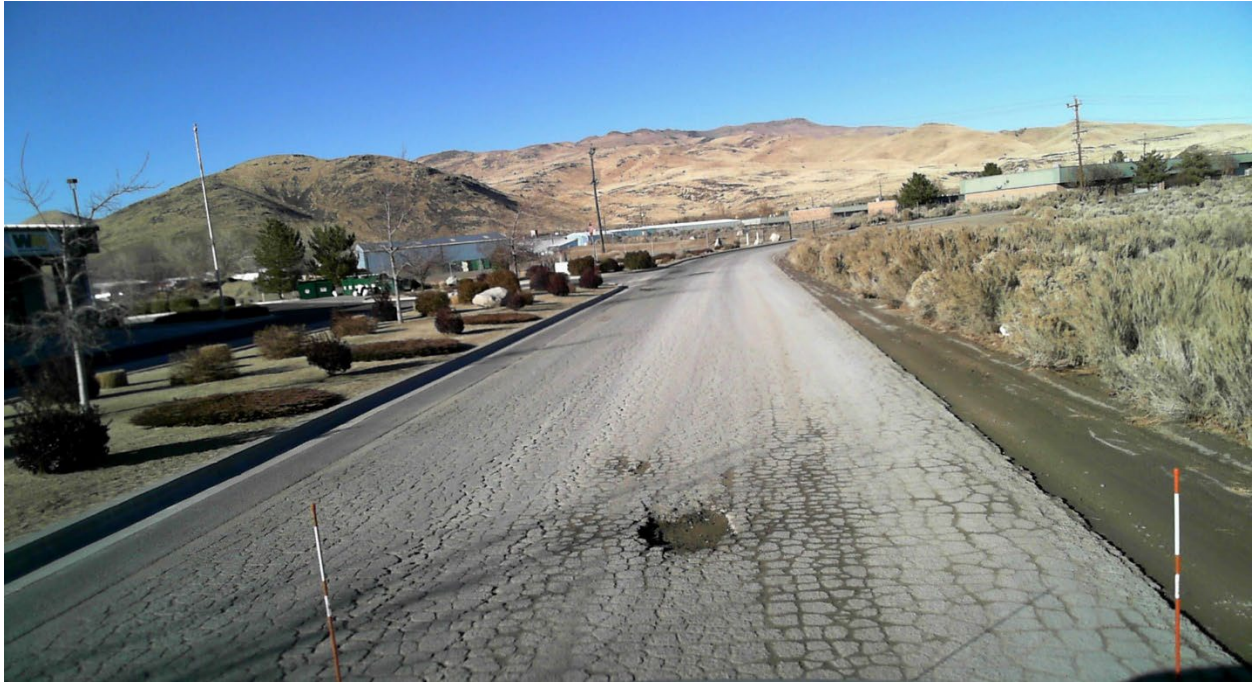
Figure 8. Pavement in Failed condition category (PCI 10-0).
