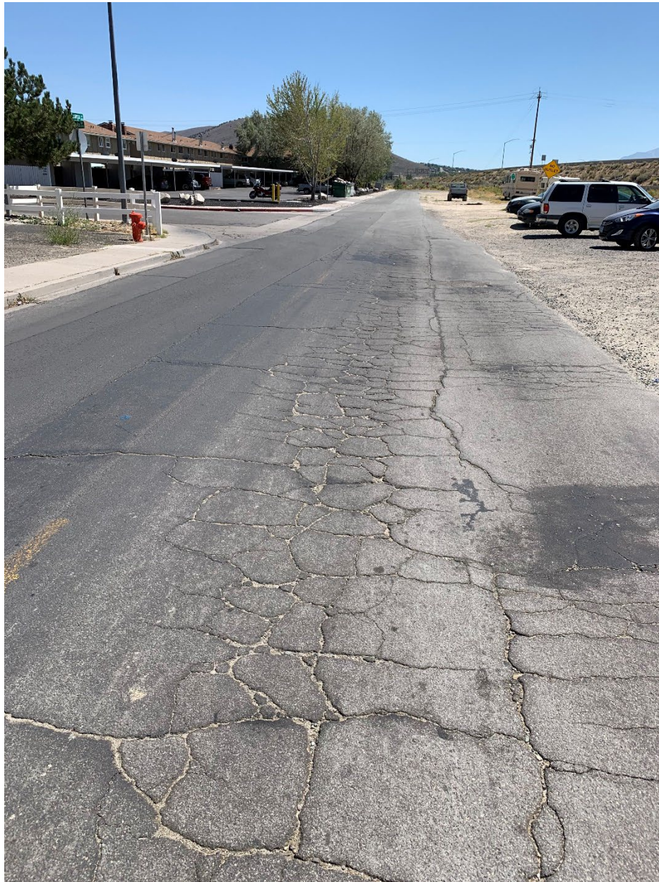
Figure 6. Pavement in Very Poor condition category (PCI 40-26).
