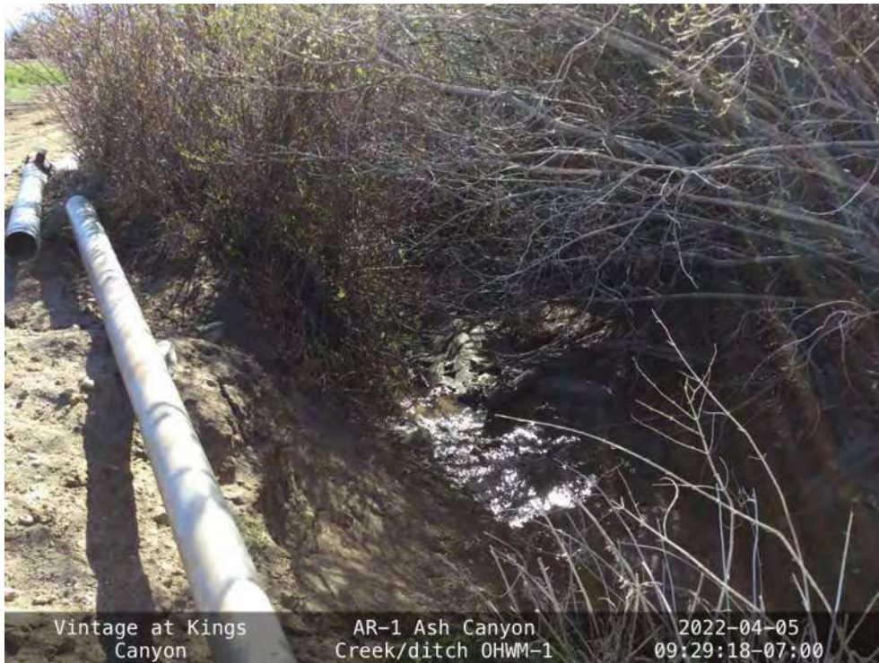
Photo 5. OHWM-1: picture showing approximately 2-4 inches of water in Ash Canyon Creek (AR-1). Exposed/partially excavated left bank with disconnected irrigation line. View looking southeast.
