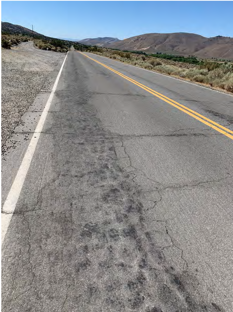
Figure 7. Pavement in Serious condition category (PCI 25-11).
