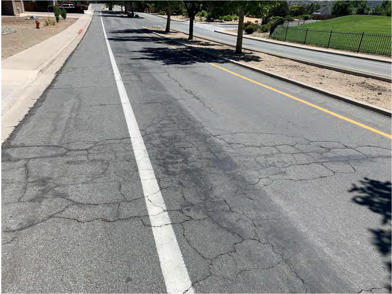
Figure 5. Pavement in Poor condition category (PCI 55-41).
