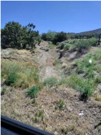
Figure 6-1. Basin forming at 2449 Pinion Hills Drive
